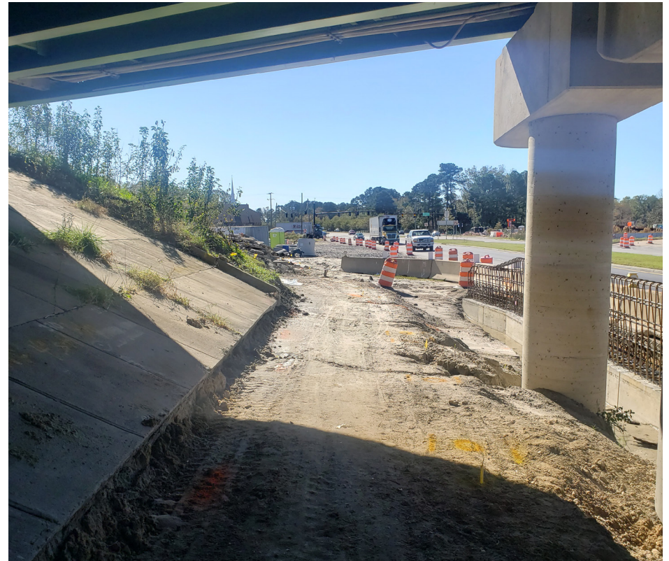
Construction of a sidepath underneath I-264 at Witchduck Road. Courtesy of Walter Camp.
