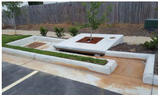
"Filterra" stormwater treatment system draining a parking lot at new suburban development site
